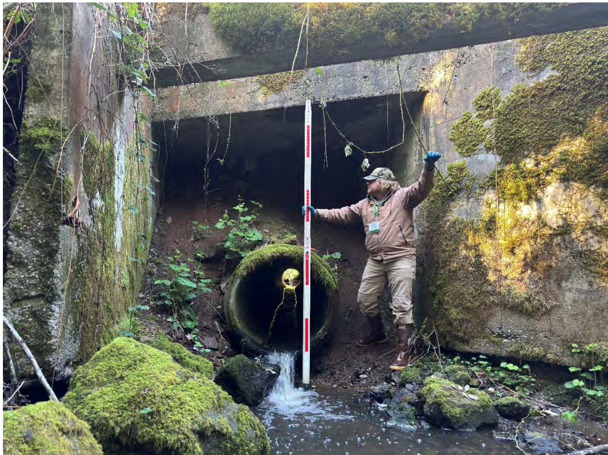
Figure 2. The downstream-most fish passage barrier culvert running under NE Country Club Road.
