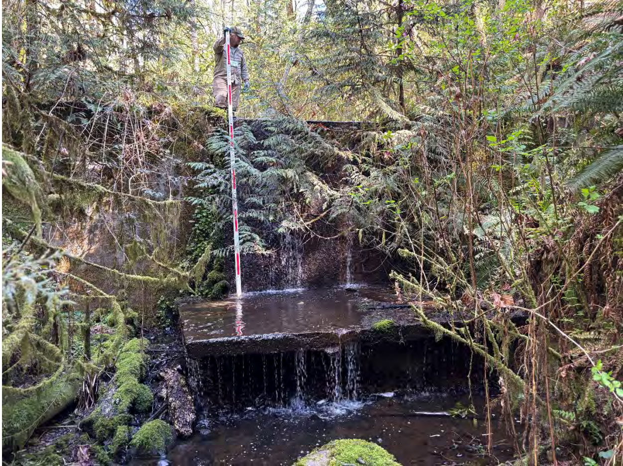
Figure 3. Derelict dam on IslandWood property.
